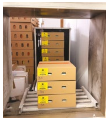
Blast freezer tunnel
